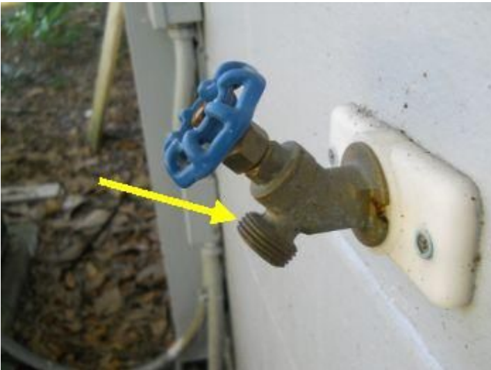
Hose bib(s) require back flow prevention
