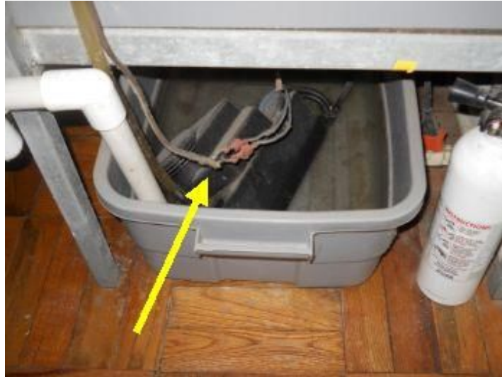
Air handler condensate pump inoperative
