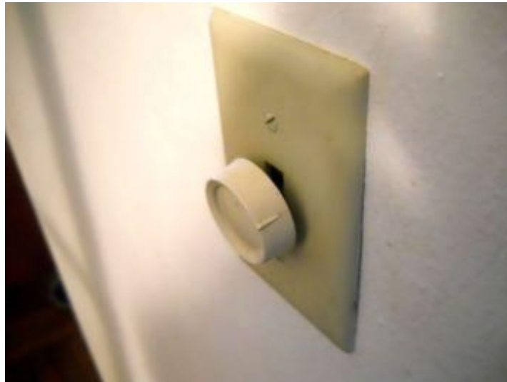
Dining room dimmer switch damaged
