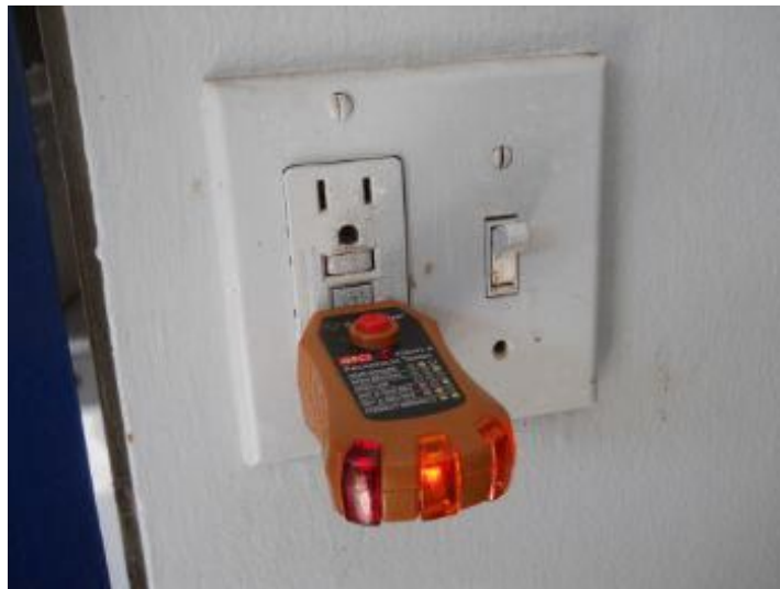
Carport GFCI outlet will not trip
