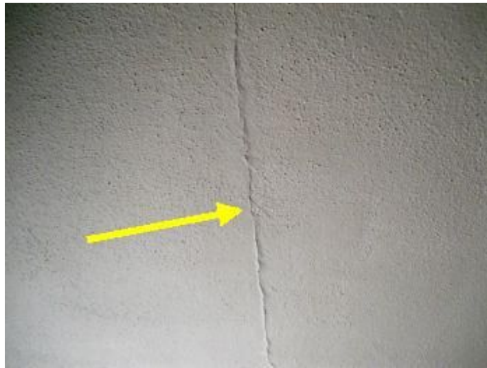
Minor ceiling damage/crack
