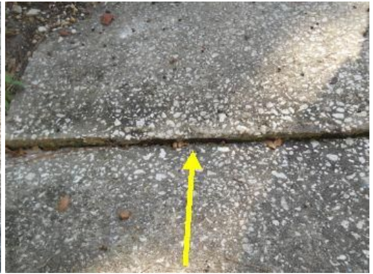
Uneven slabs.... Tripping hazard at driveway
