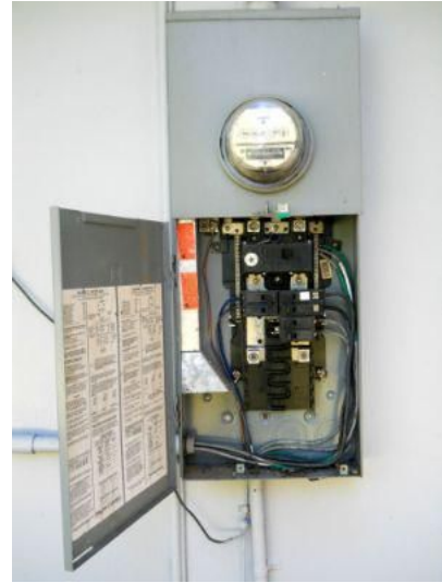
Square D 200 amp service main open for inspection
