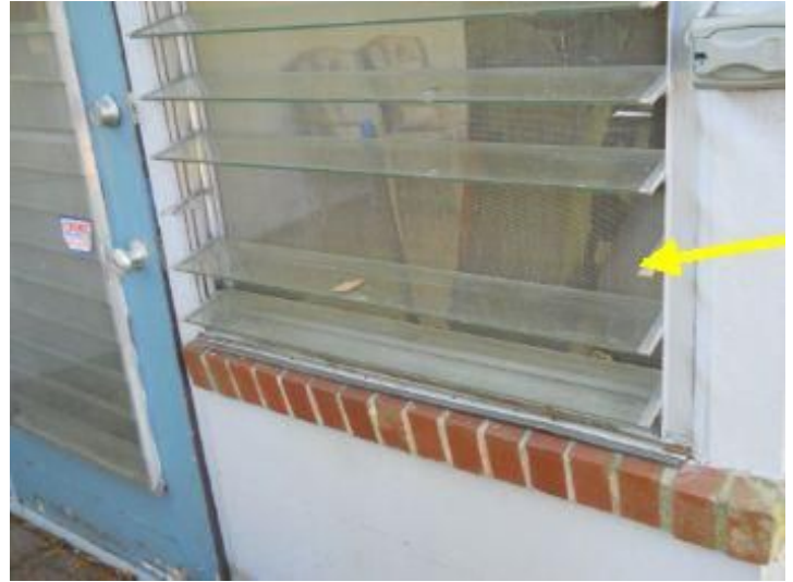
Two jalousie panes missing
