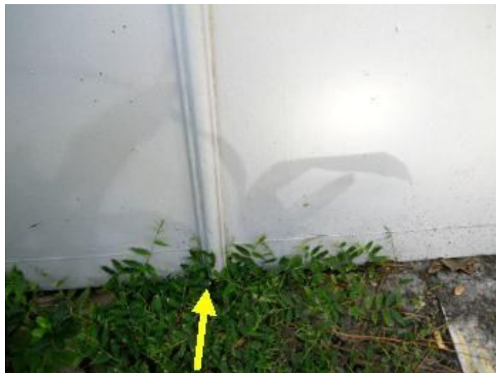
Siding to soil contact
