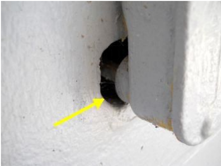
All exterior openings need sealing
