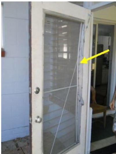
Florida room door screen damaged
