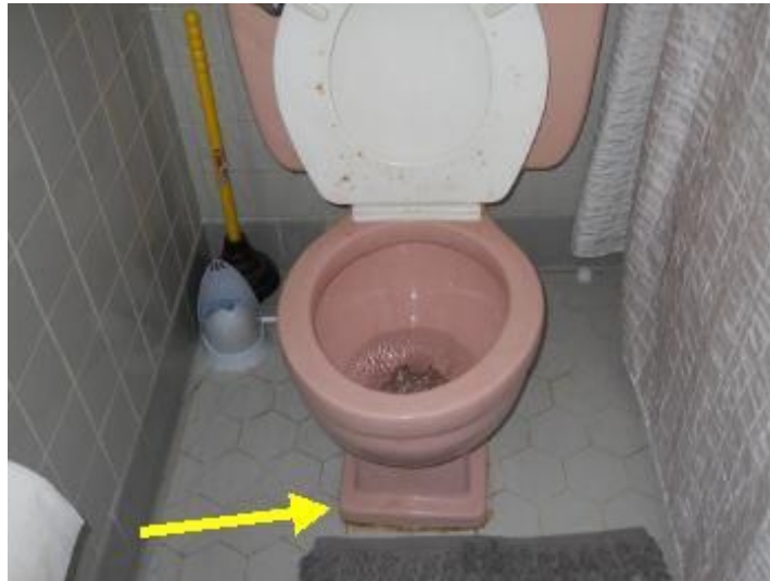
Guest bath toilet loose at floor
