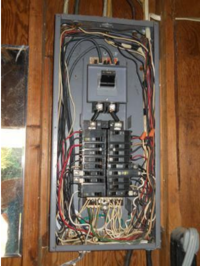
Square D 100 amp service sub open for inspection
