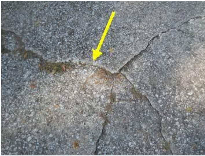
Extensive cracking at driveway
