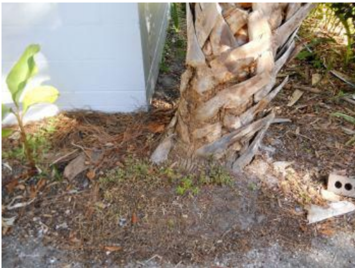
Tree close to the foundation
