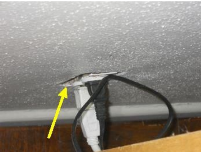
Bedroom #2 cover plate missing
