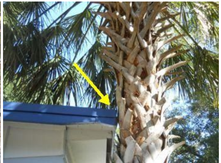
Tree close to the fascia
