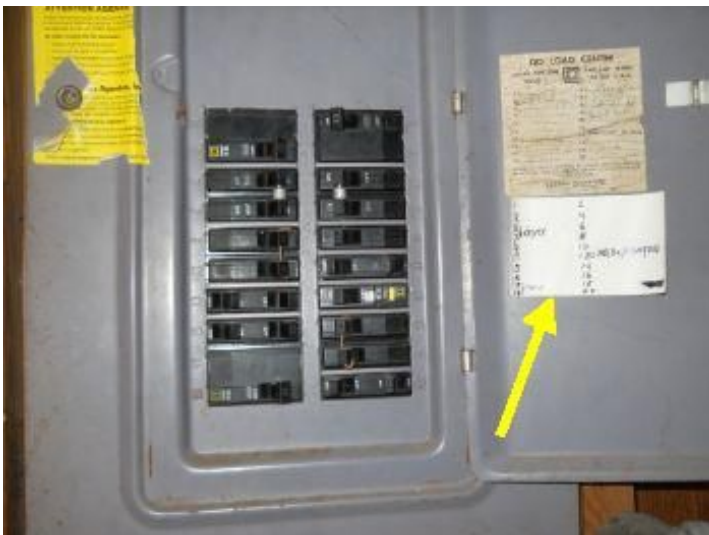
Breaker(s) need proper labeling
