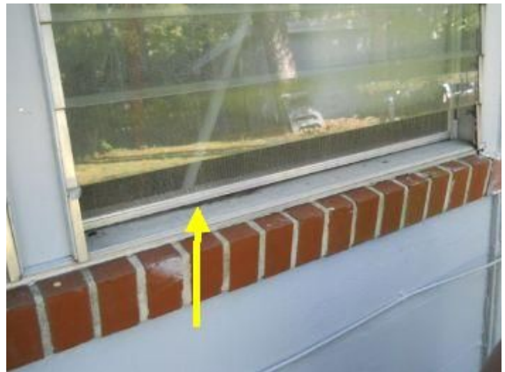
Two jalousie panes missing
