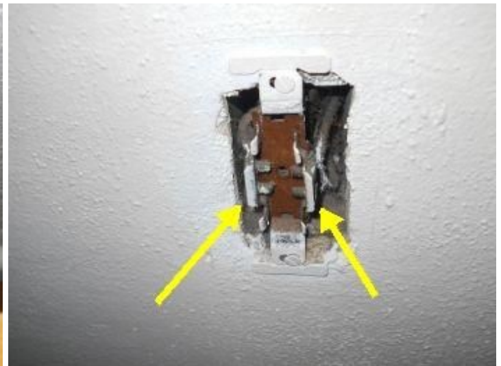
Bedroom #1 outlet damaged... Electrocution hazard
