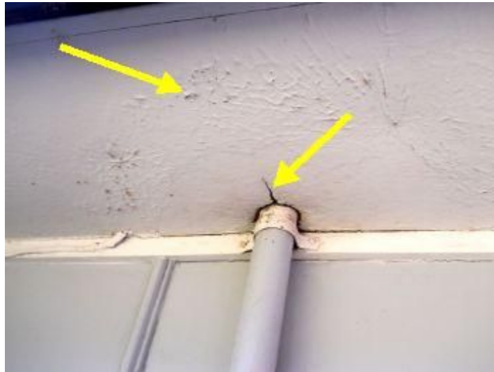
Moisture damage at power mast
