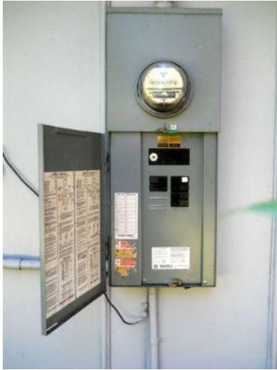
Square D 200 amp service main
