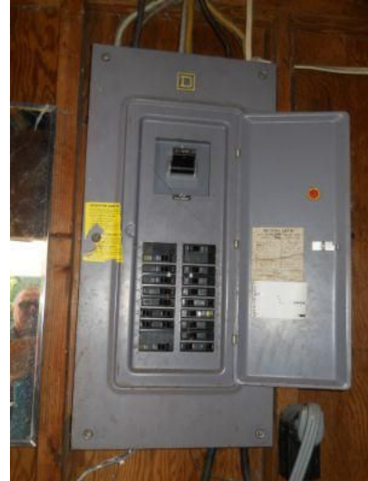
Square D 100 amp service sub
