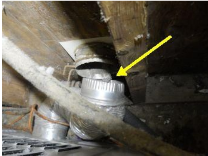
Clothes dryer duct loose
