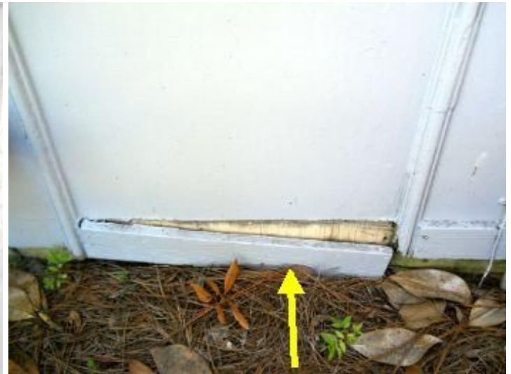
Loose trim West elevation
